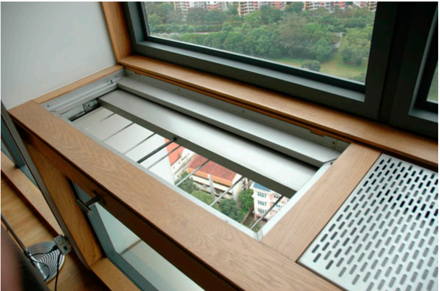
Figure 6: Monsoon window at One Moulmein Rise, Singapore, with slideable panel to regulate airflow. Ventana para el monsoon, con sistema regulable para el flujo de aire.
